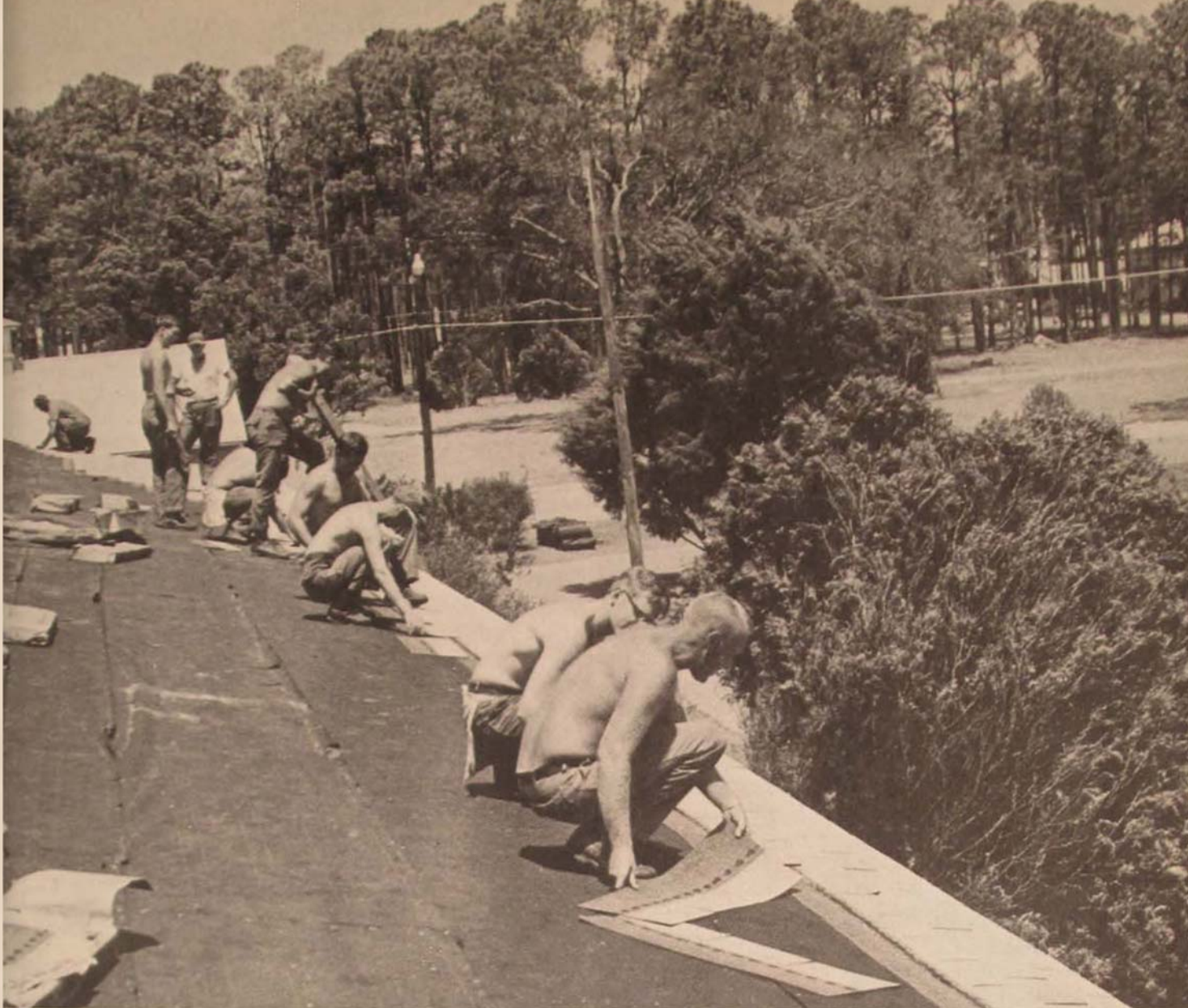
Prime BEEF crew repairs damage from Hurricane Camille at Keesler AFB, Mississippi.
