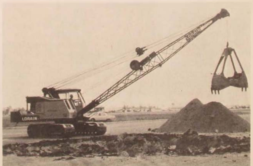
HORSE heavy equipment, in tests at Eglin Florida, proves ability to repair bomb damage.
